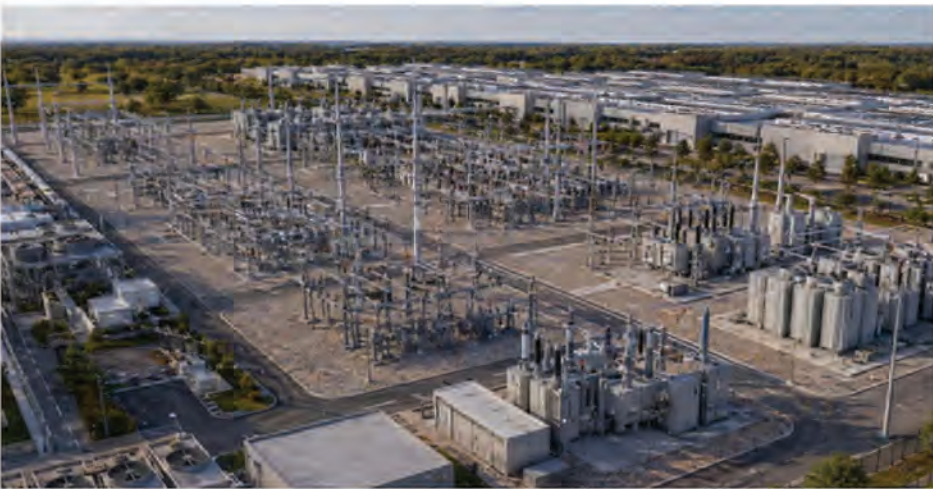
Substation and Switchyard - Ashburn, VA, 110 Megawatts
