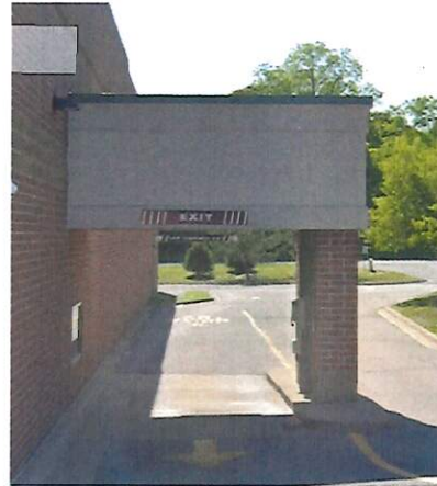
EXISTING SCOPE OF WORK: PHARMACY CANOPY - REMOVE AND INSTALL NEW ENTER LETTER SET.
