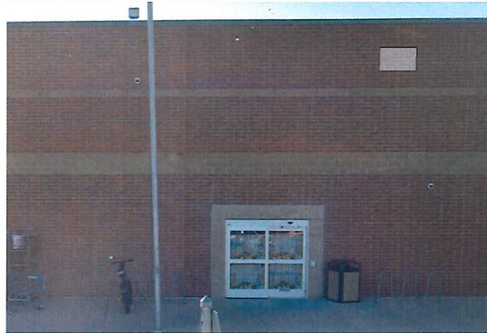
EXISTING SCOPE OF WORK: FRONT ELEVATION - REMOVE AND INSTALL NEW WHITE PHARMACY LETTERSET.
