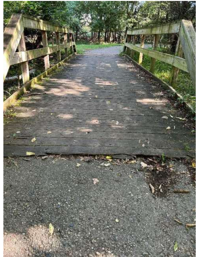
Settlement at Bridge Approach
