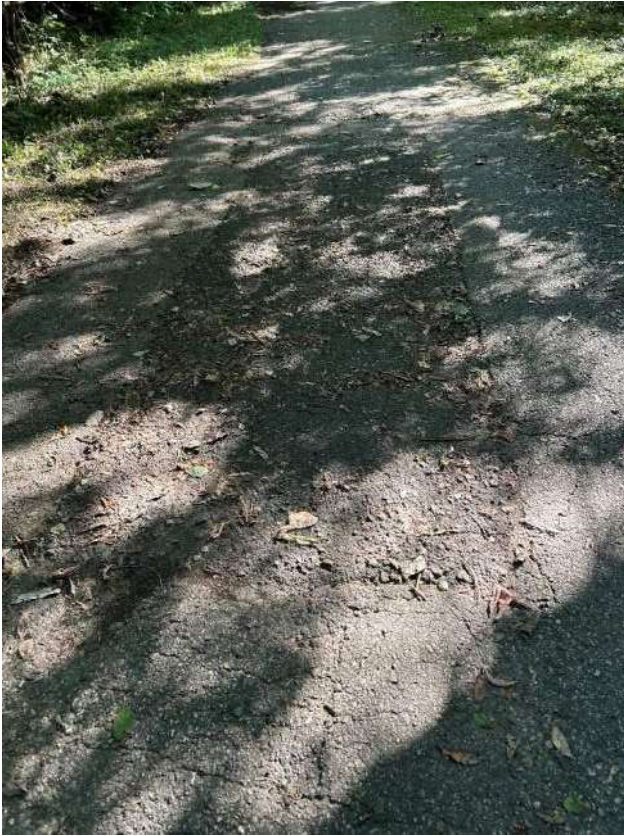
Deteriorated Asphalt Patch
