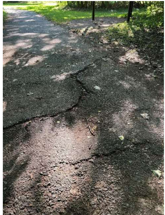
HMA Path Heaving and Cracking
