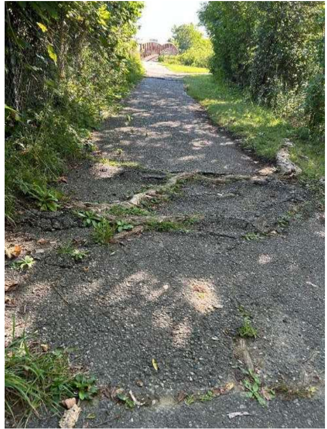
Root-Related Pavement Heaving; Point of End
