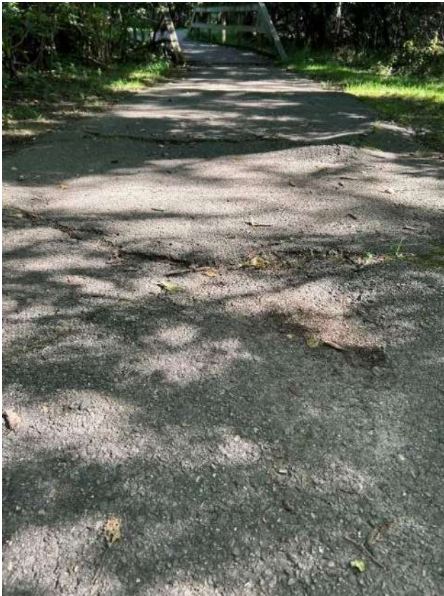
HMA Path Heaving and Cracking
