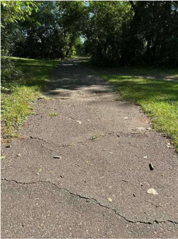
HMA Path Heaving and Cracking
