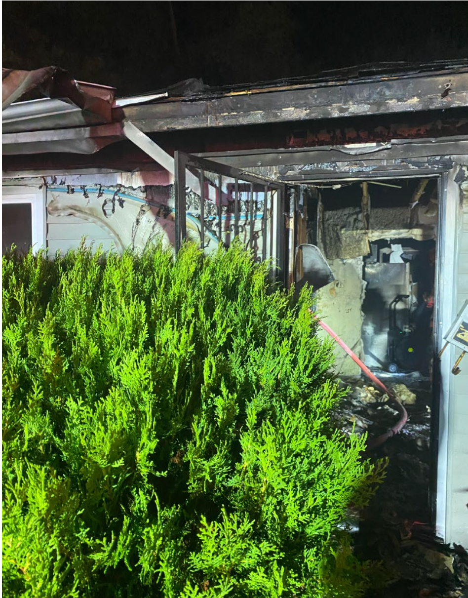
Exterior photo by YTFD following the fire.
