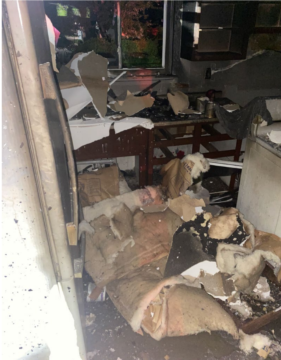
Interior photo by YTFD following the fire.
