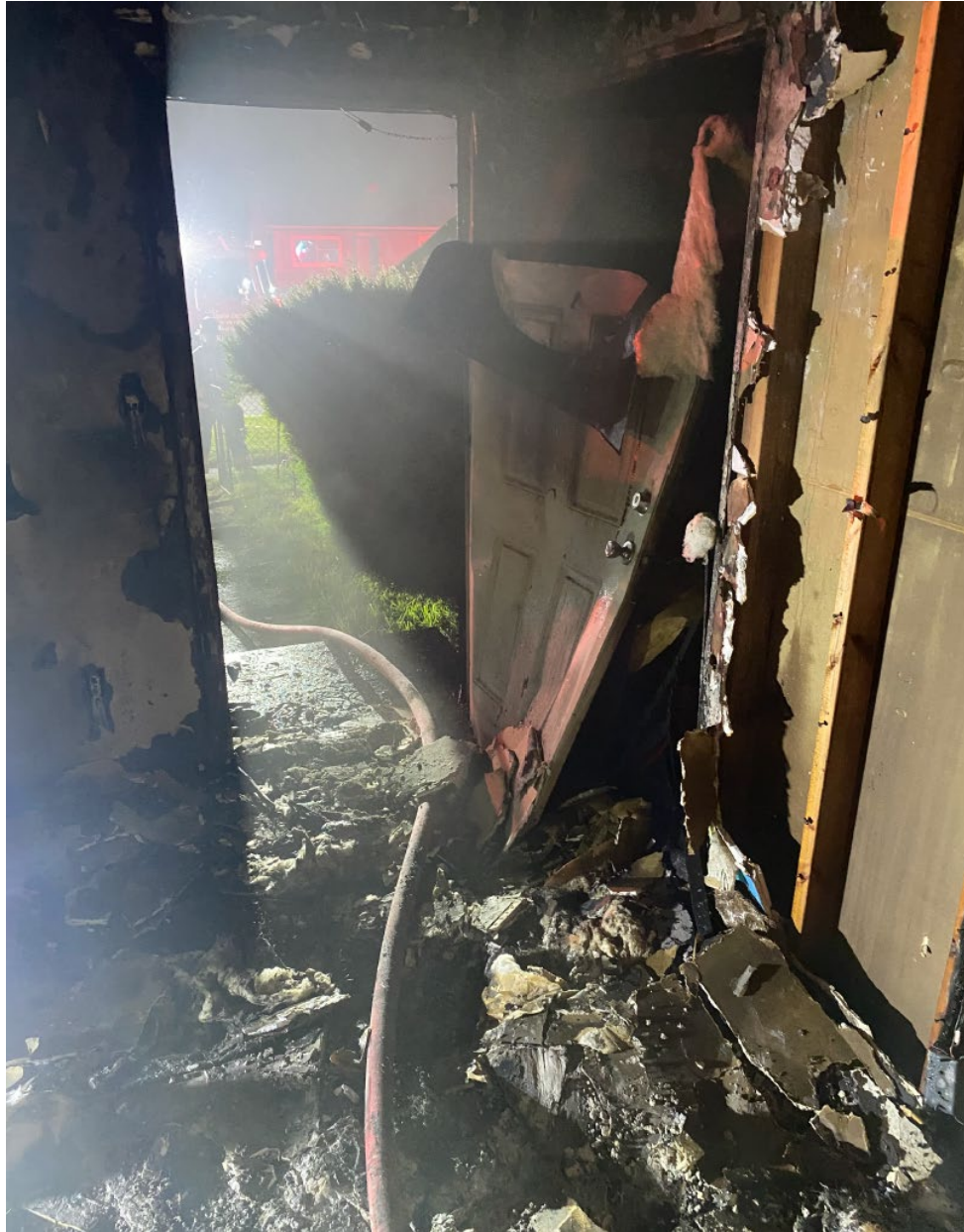
Interior photo by YTFD following the fire.
