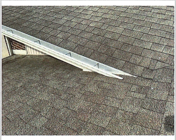
Open gutter should be capped to prevent large volume of water rushing behind flashing.
