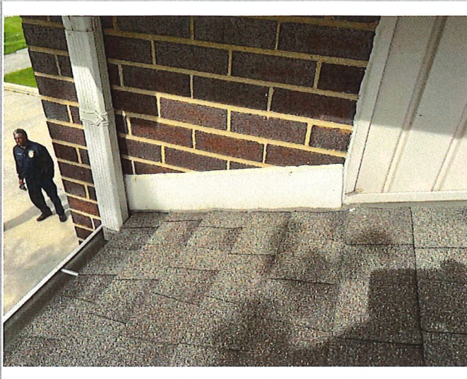
Counter flashing not cut into brick, manufacturer requires reglet (cut into brick)
