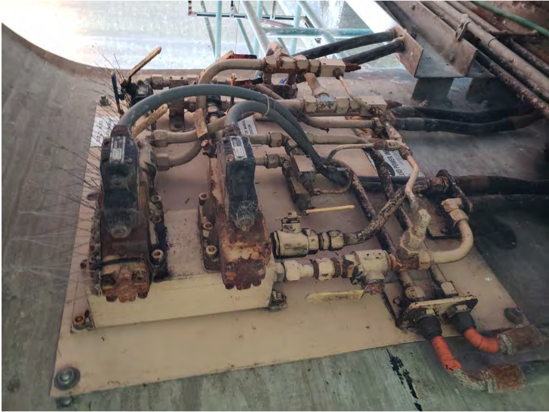
Picture of Gate Controls
