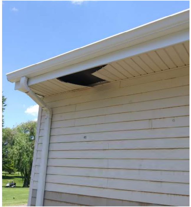
Exterior 52 Broken Soffit Side B
