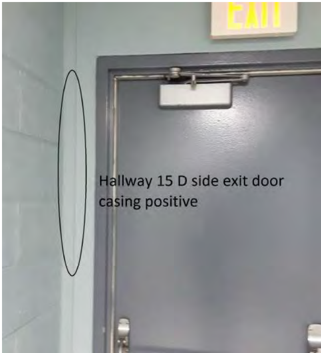
Hallway 15 Exit door Casing Positive
