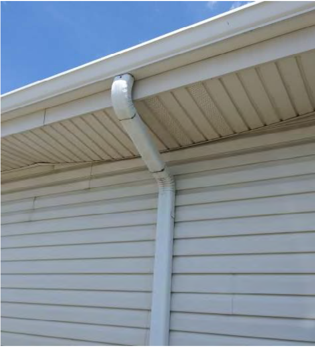
Exterior 52 Broken Soffit Side A
