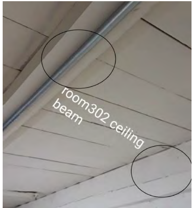
Room 302 Ceiling Beams Positive
