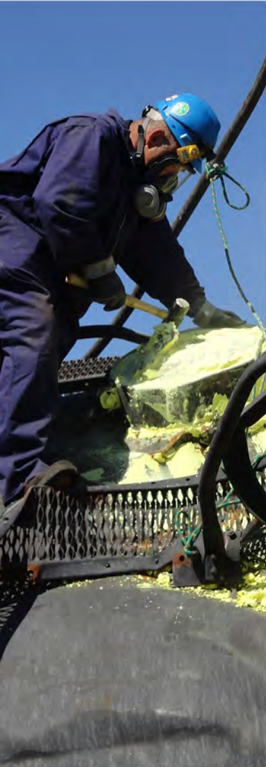
USE PERSONNEL WORKING ON DAMAGED RAIL CAR FROM DERAILMENT IN LIGONIER INDIANA
