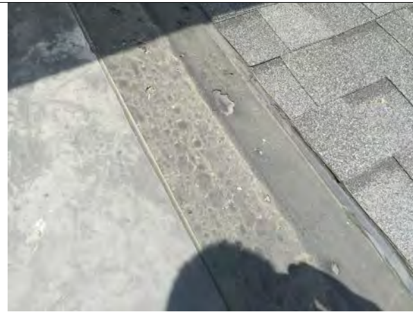
The flashing membrane utilized to join these two roof sections has failed and will require replacement.
