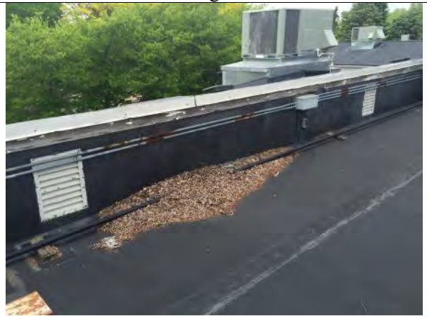
Debris / Parapet Wall / Nailer Deterioration – Several small corrections will need to be made to ensure this detail is water-tight.
