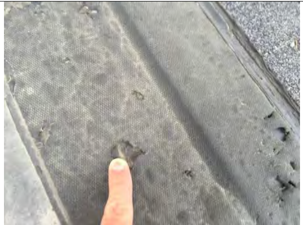
Premature flashing failure between two roof sections was noted throughout.
