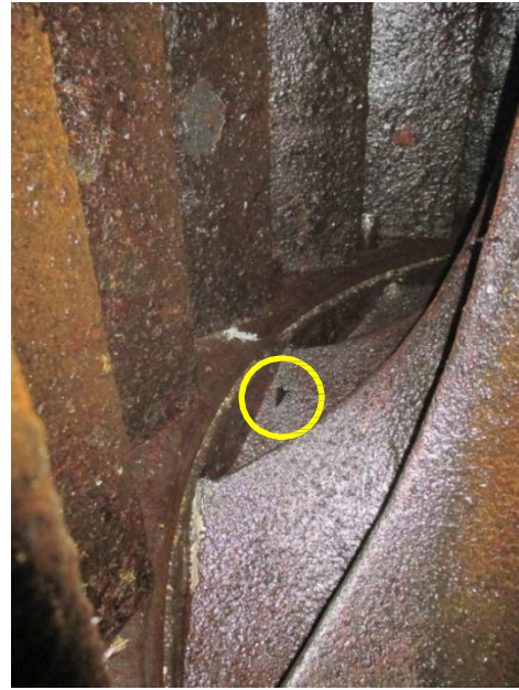
Runner- showing 1 of 2 holes in the buckets
