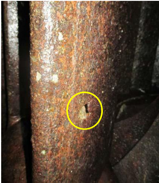
Wicket Gate- showing a hole in the outer membrane
