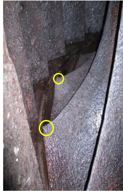
Runner- showing 2 of multiple cracks in bucket
