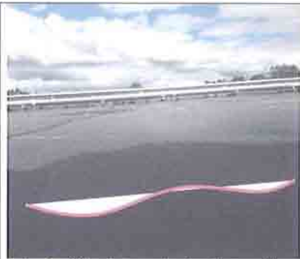
Adhesion failure between the first & second layer of insulation has caused the insulation to curl
