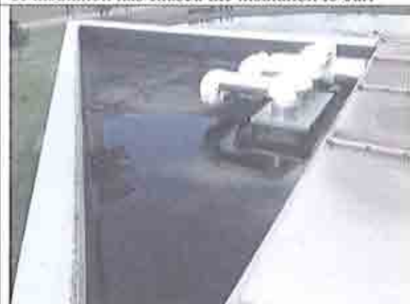
Poor drainage, ponding water after four dry days
