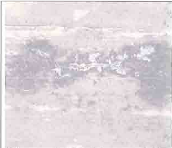
Moisture traveling through the concrete decking
