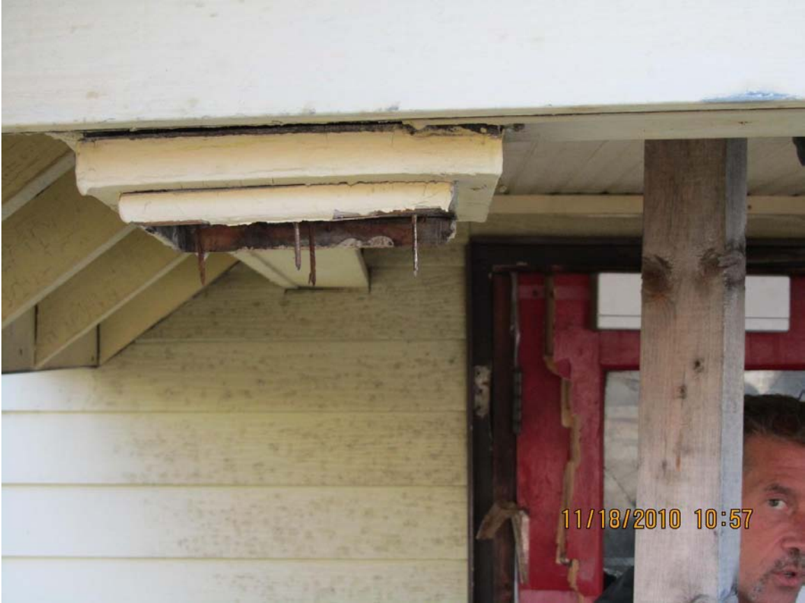
TOP PORTION OF BROKEN PORCH COLUMN
