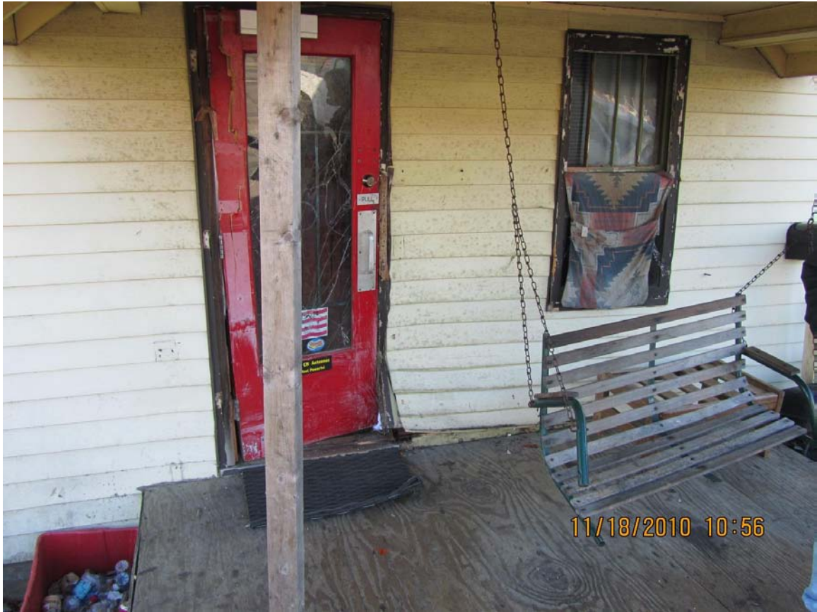
FRONT DOOR, WALL AND PORCH COLUMN SEVERELY DAMAGED AND IS FAILING
