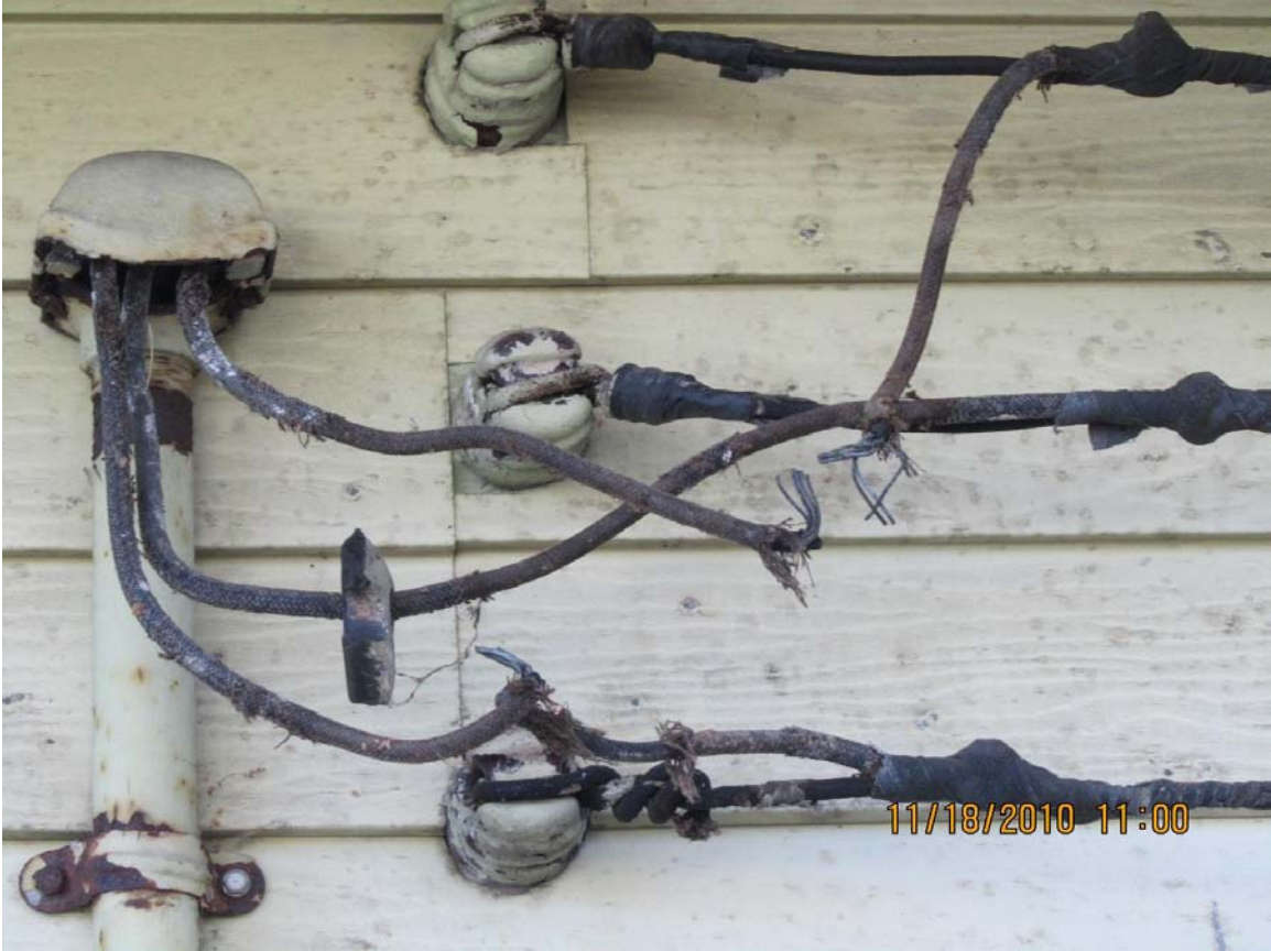
DISCONNECTED ELECTRICAL DTE WIRES
