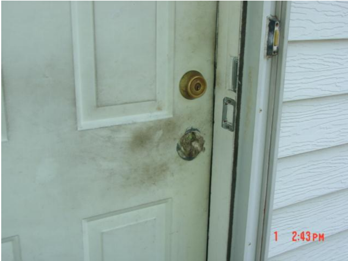
MISSING HANDSET WHICH MUST BE REPLACED AND/OR REINSTALLED
