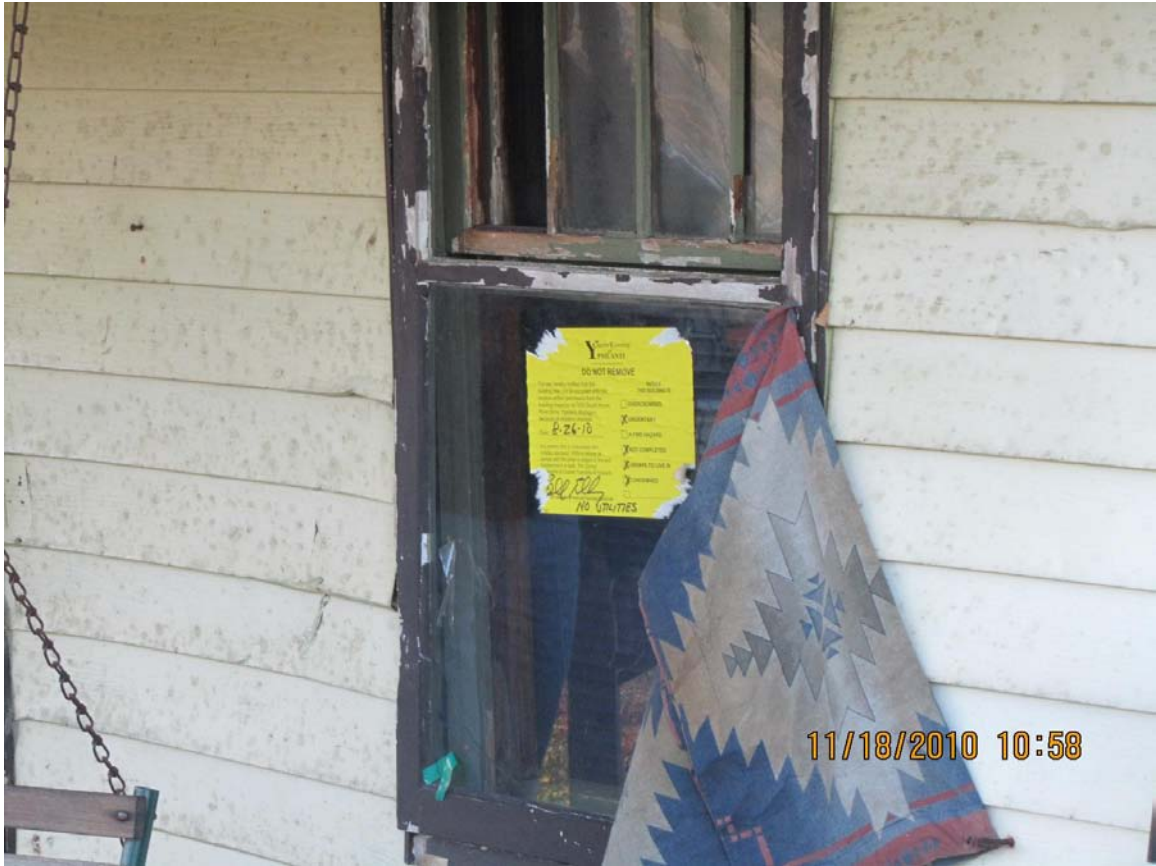
ORIGINAL CONDEMNATION PLACARD WHICH WAS AFFIXED TO THE FRONT WINDOW ON 08-26-2010
