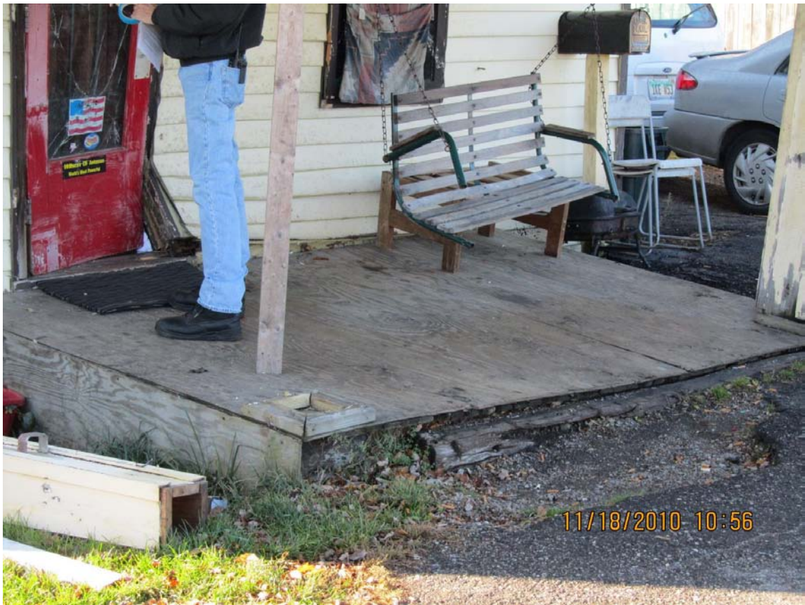
FRONT PORCH IS ROTTED AND HAS COLLAPSED
