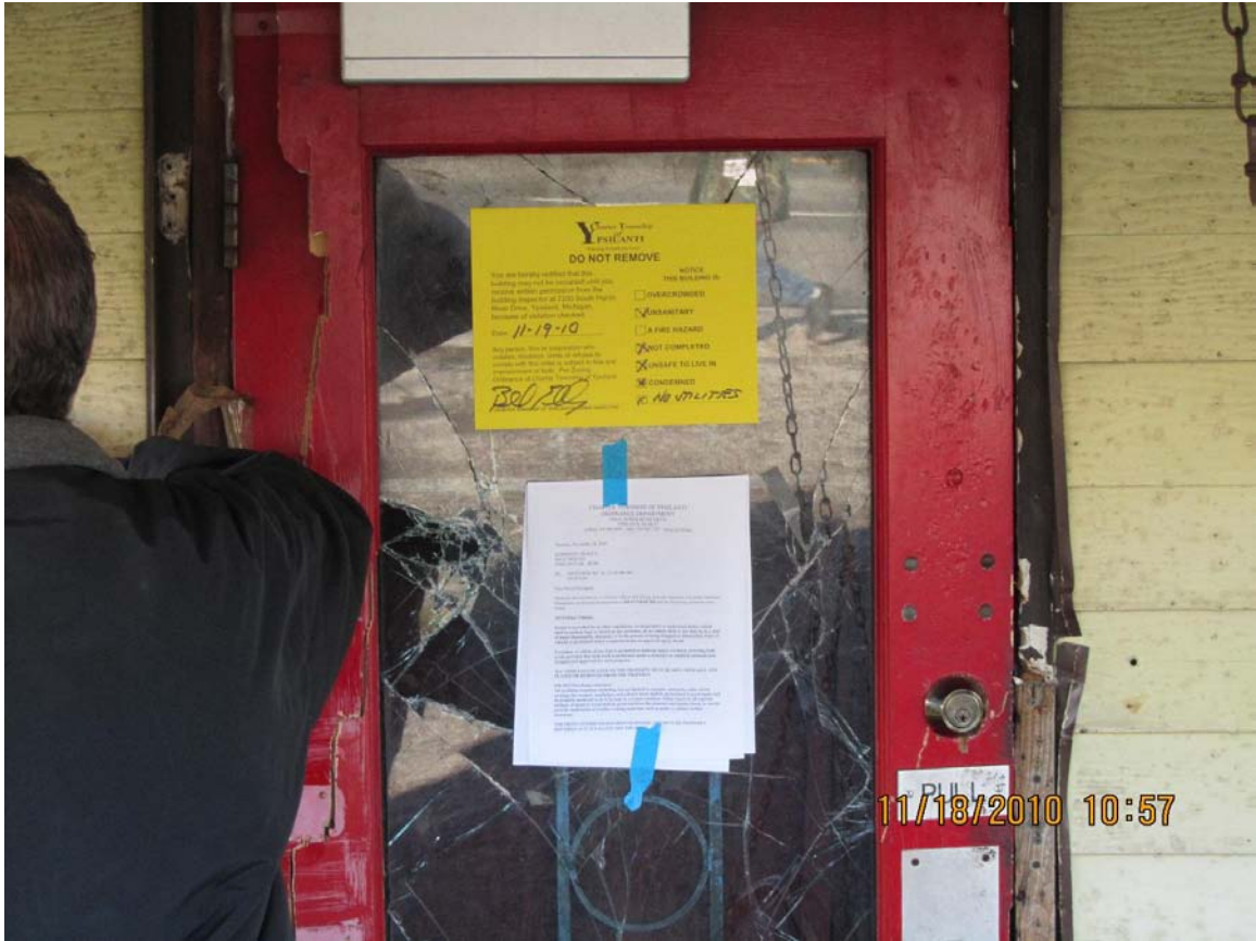
DAMAGED FRONT DOOR/FRONT WALL. CONDEMNATION PLACARD AFFIXED TO FRONT ENTRANCE DOOR
