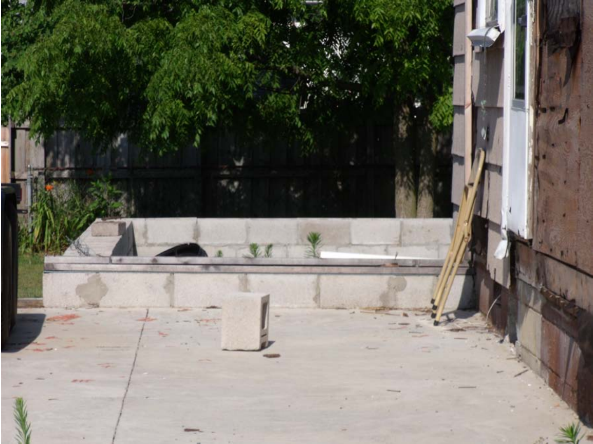
Photo #2, 3 & 4: Foundation of addition on rear of home and garage slab. Work ceased on addition October of 2007
