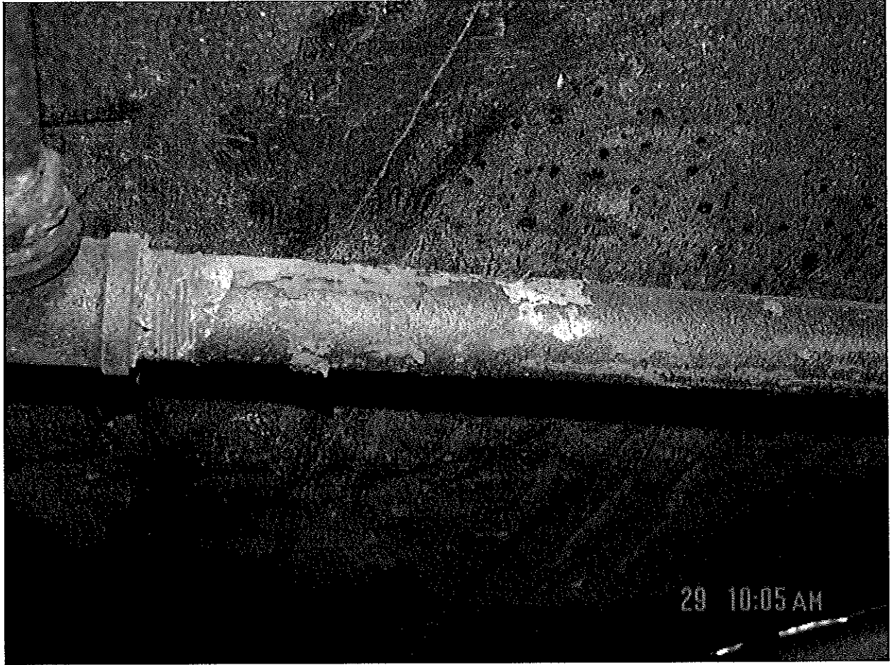
Rusted/corroded gas line located in basement/crawlspace area
