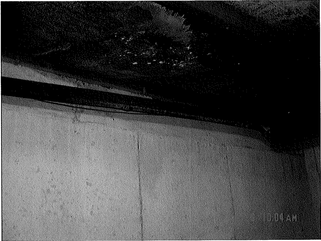
Bent and twisted metal support frame located in the basement/crawlspace
