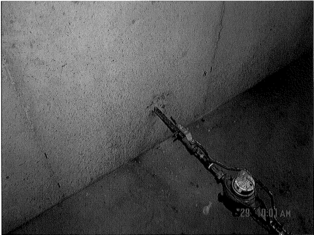
Main water supply line which is required to have a sleeve installed over the copper water line and through the concrete wall
